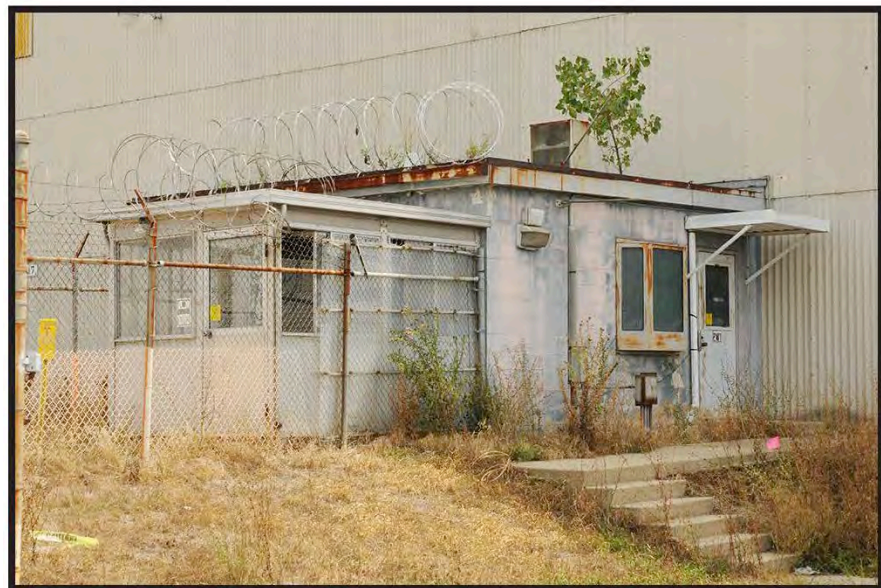
Figure 5: North Side of the X-111B Special Nuclear Materials Monitoring Portal, August 2014, Facing Southeast
