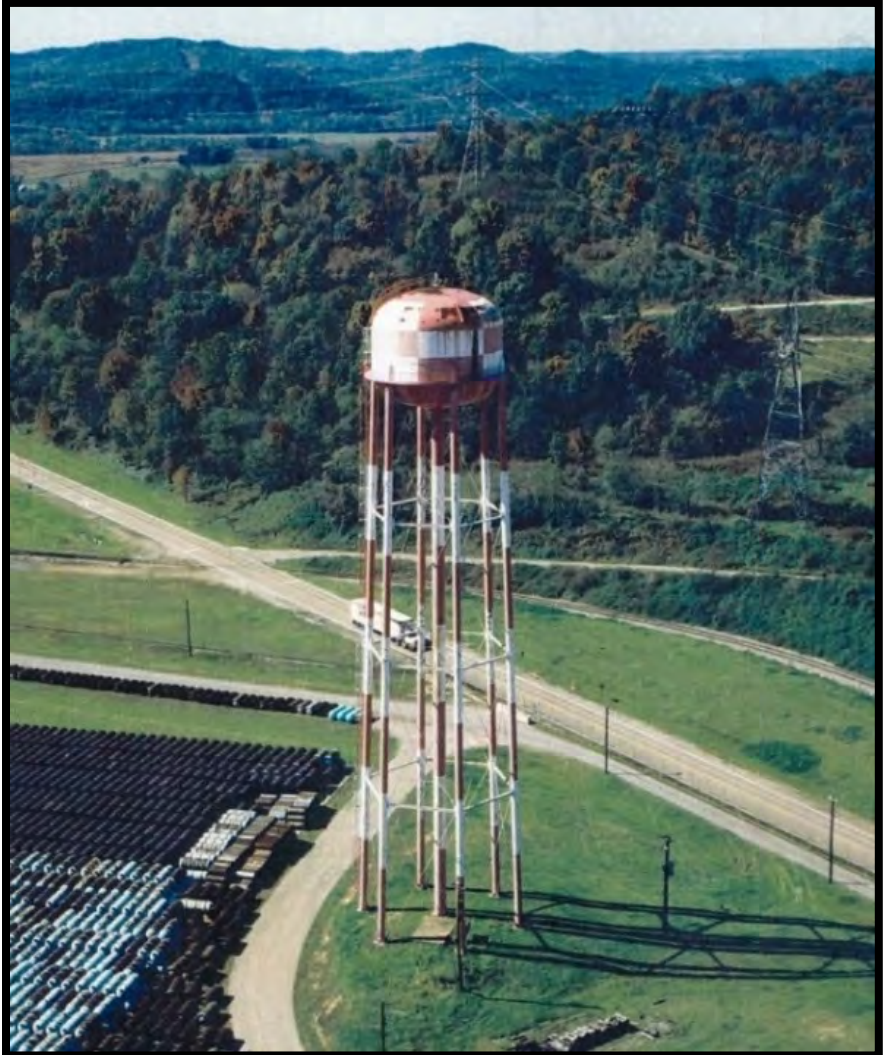
Figure 2: Northeast Side of the X-612 Elevated Water Tank, Facing Southwest (ca. 1980s)
