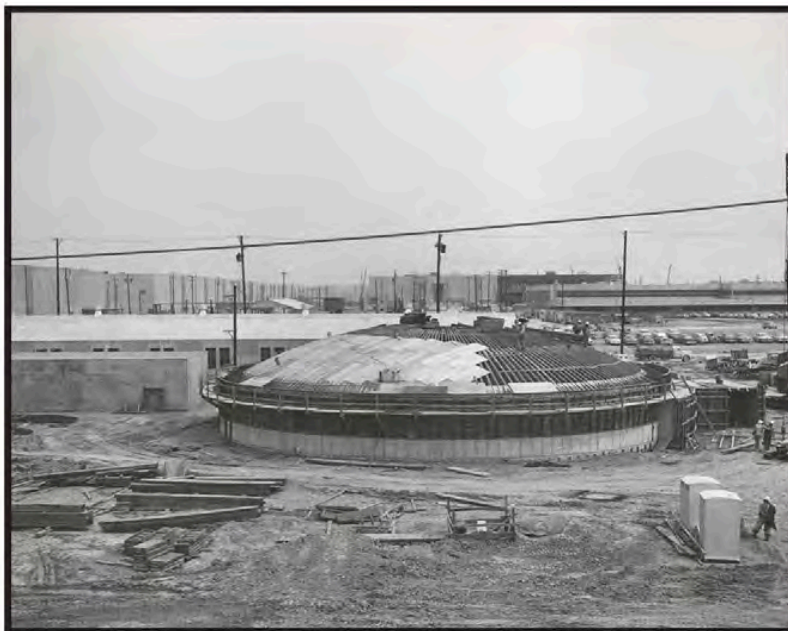
Figure 6: X-300A Process Monitoring Building, X-300 Plant Control Facility Under Construction to Right of X-300A, May 1954
