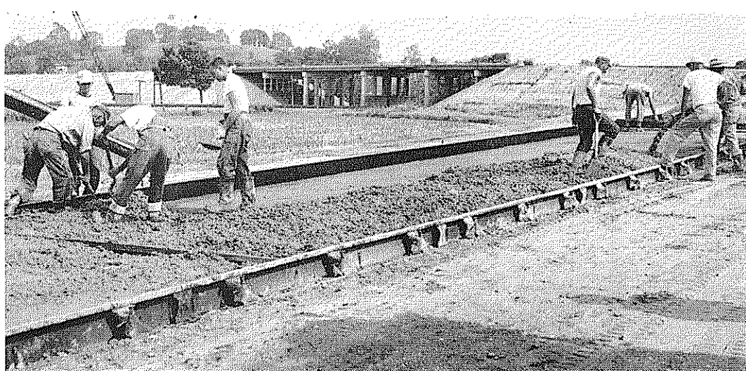
OVERPASS ROAD TO A-PLANT NEARS COMPLETION. Highway contractors are shown finishing the pouring of concrete on the overpass road leading into the A-plant. The picture was taken looking south. The over-
