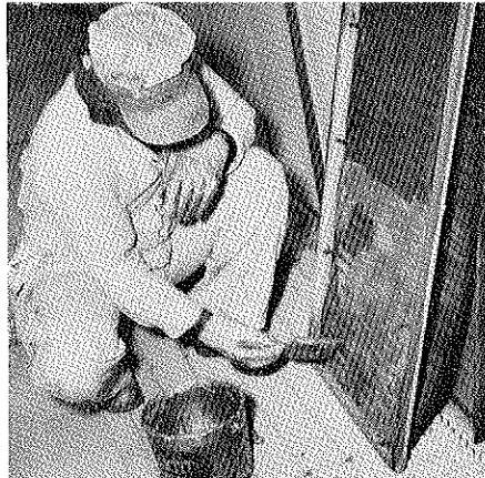
FINISHING TOUCHES. Earl Jordan, paint shop, is one of those responsible for securing the huge cubicles from the ravages of the elements.
