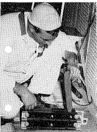
As the old wooden operating rods are replaced, the new resin rod assembly is being installed by Earl Williams.
