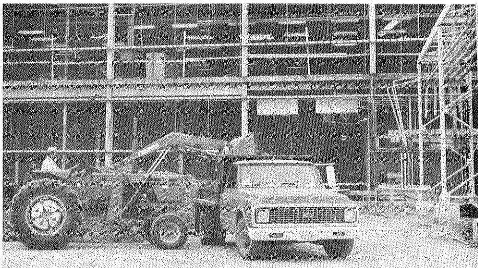
Restoration work is underway on X-344 Building to be used as UF6 weighing and sampling facility.
