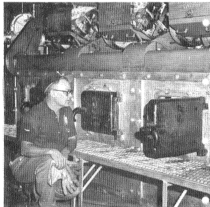
THE FIRE IN NO. 2 coal stoker is being inspected by Jim Keesee, station engineer.
