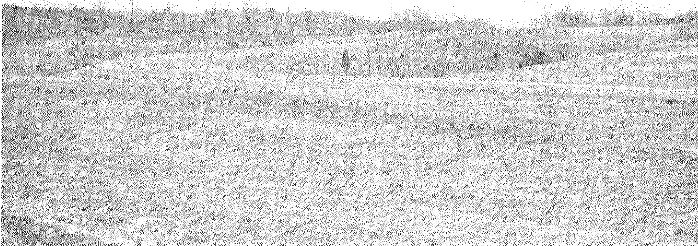
Preparation work for the new south perimeter road was completed ahead of schedule last fall. Paving operations will begin within the next few weeks. Department of Energy officials now predict a mid-summer opening for the new road. Completion originally was scheduled for November of 1979.
