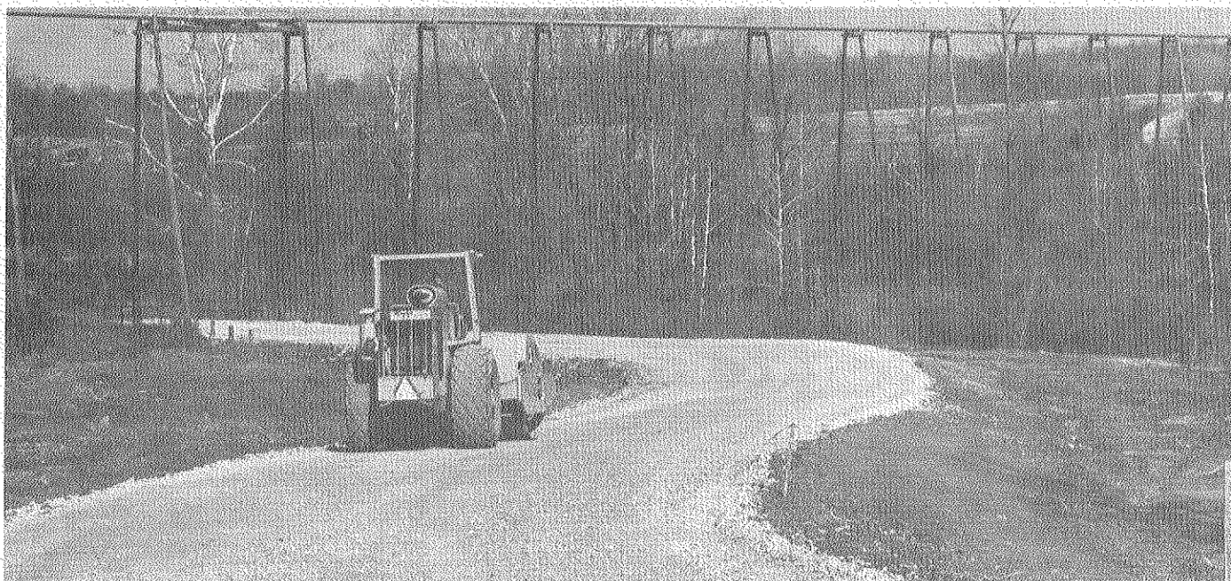
Construction work now is under way to reactivate and improve an old access road which connects the east and north arteries into the plant complex. The road is being used by residents to the east of the plant, who have been inconvenienced and using unimproved gravel roads for access to their area. The strike of OCAW Local 3-689 and resulting closing of the north and east access roads have prohibited their use since May 3. Paving is to be completed in the spring. The road is expected to be utilized in the future as a bypass route for plant traffic which must be detoured because of cooling tower fog conditions.
